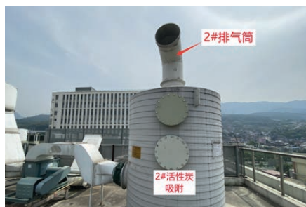
▶ 屋顶增设的活性炭吸附塔
